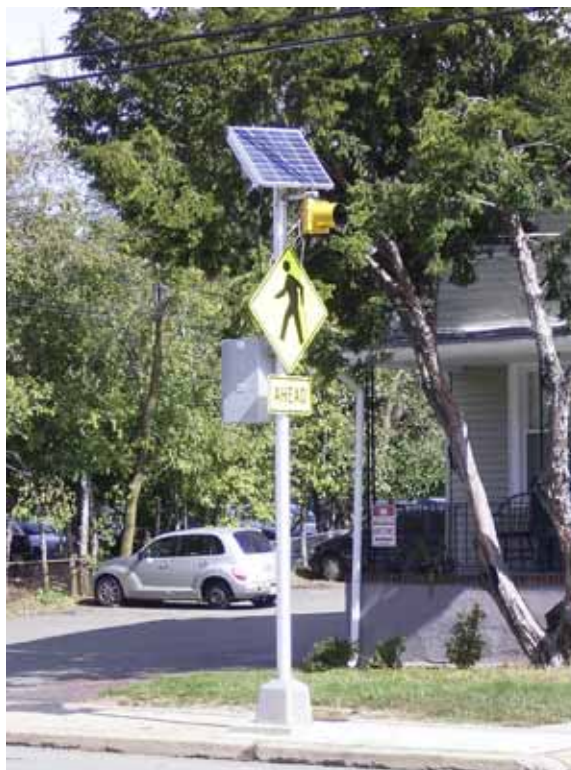
Solar-Powered Pedestrian Signals
